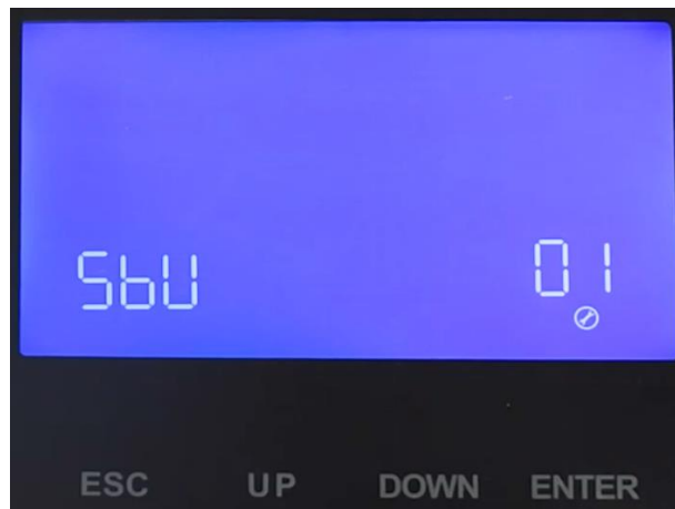
Figure 2.1.5.6 Growatt operation panel
