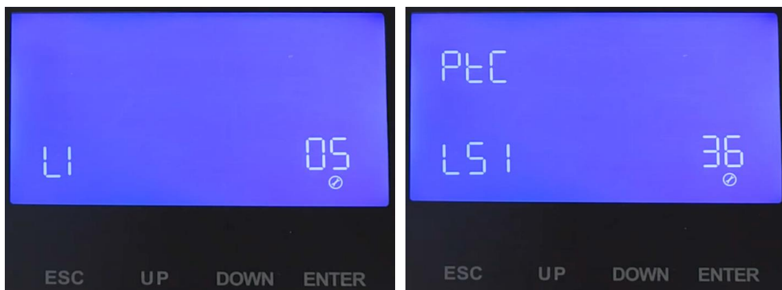
Figure 2.1.5.9 Growatt operation panel
